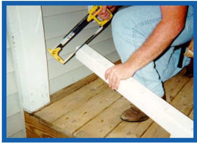
STEP 2: Trim each side of top and bottom rail equally to assure uniform appearance upon completion.
